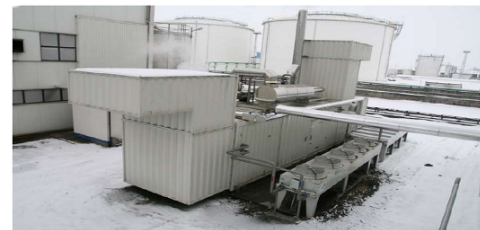
Fig. 51. View of a cogeneration system with an electrical output of 1.5MW and a thermal output of 1.7MW
