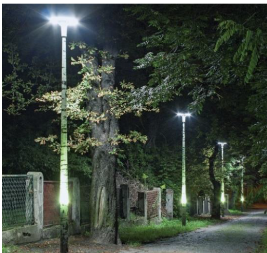
Fig. 45. Implementation of lighting on composite poles with birch graphics illuminated by an internal additional light source. Pabianice, Lewityn MOSIR
